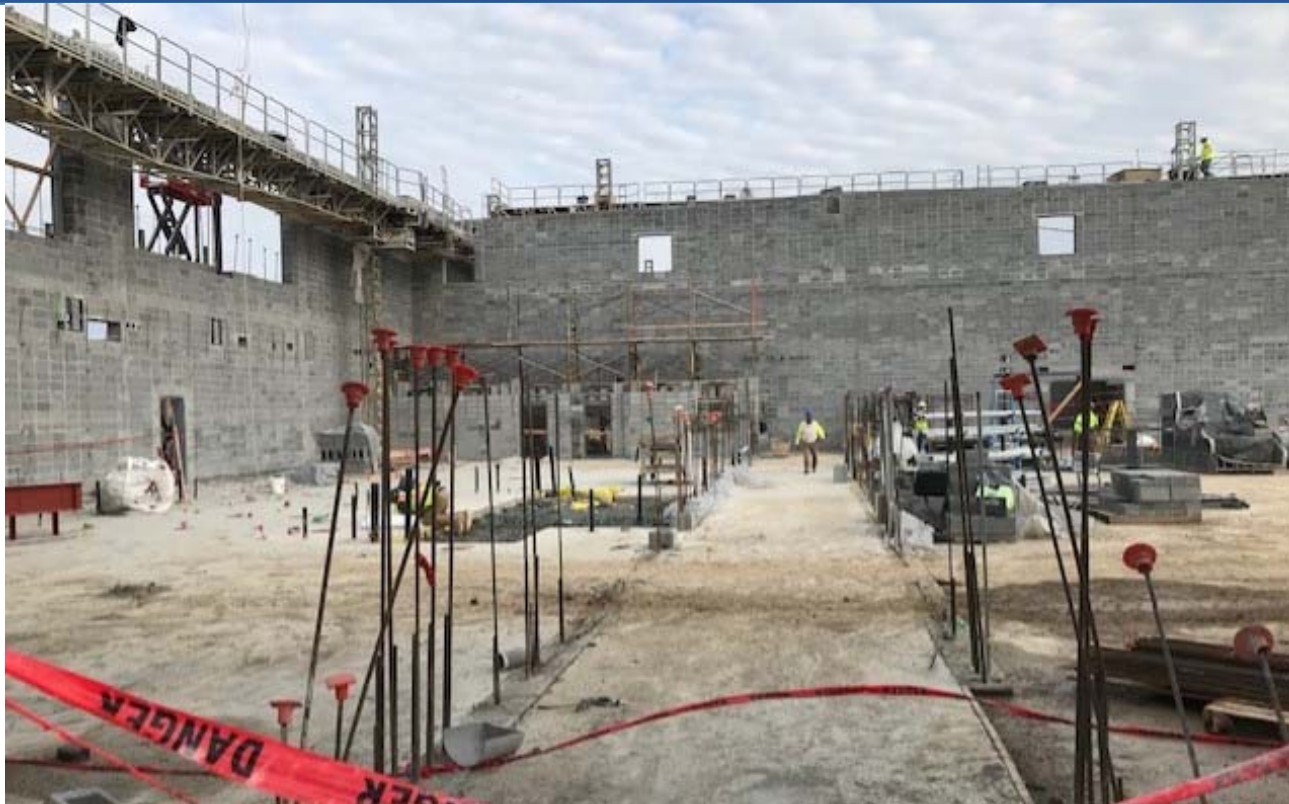
View of interior athletic corridor, locker rooms on left, Aux gym on right
