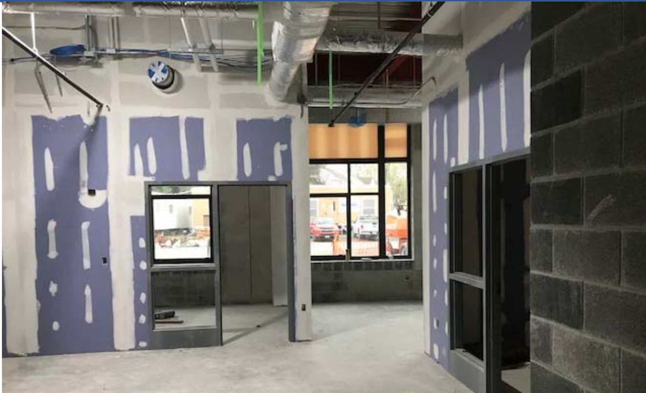
Interior of the new health suite with wall installation
