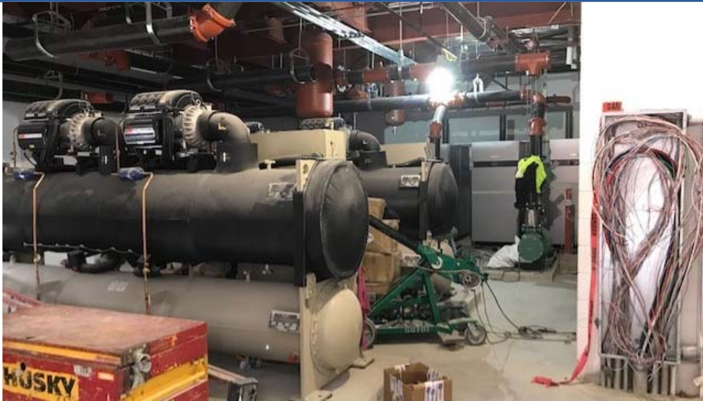
Mechanical room with boilers and equipment installed
